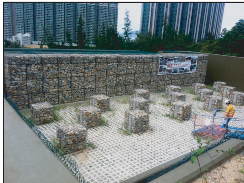
Figure 2. Baffles installed upstream of the rigid barrier on Lantau Island, Hong Kong.[5]
