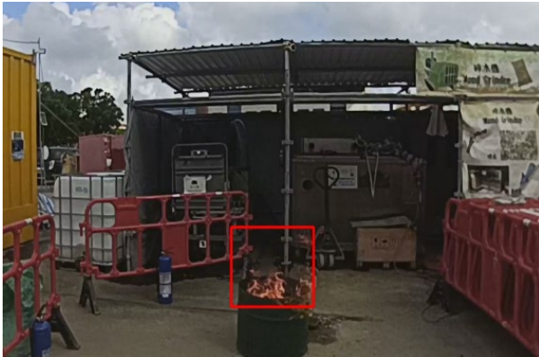
Figure 7. Successful detection of fire at a worksite during the trial.
