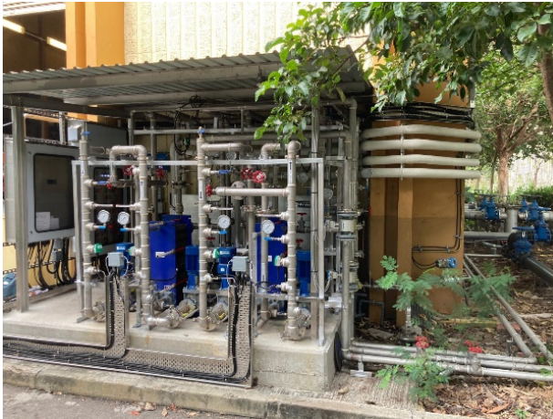
Figure 4. Pilot effluent cooling A/C system at the Sha Tin STW.
