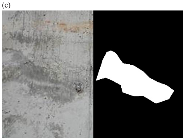
Figure 4. Data labelling for the micro inspection of (a) cracks; (b) delamination; and (c) stains.
