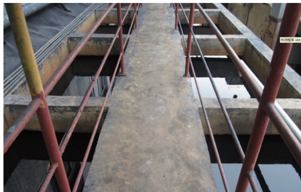
Figure 13. Denim Factory 'C' WWTP, Shenzhen, Guangdong, PRC.
