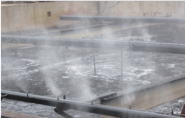
Figure 7. MNT dosing application in WWTP.
